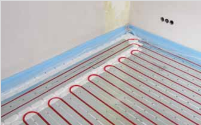
Completed heating system TS
